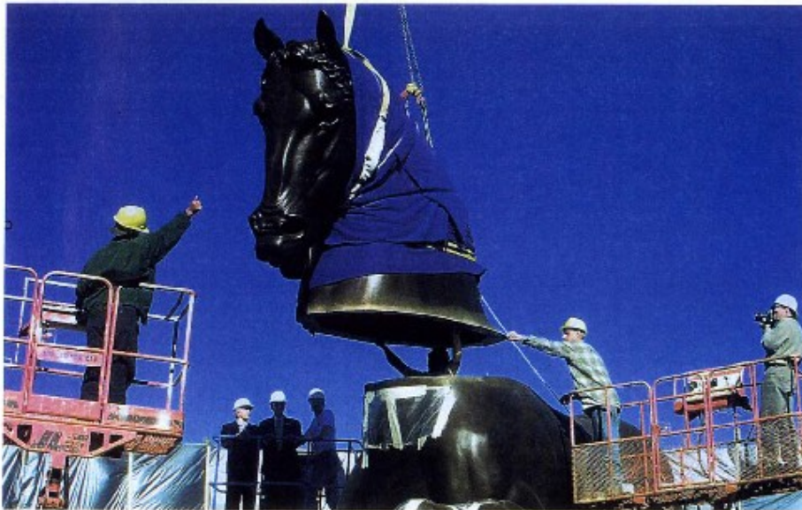
Craftsmen from the Tallix Art Foundry in Beacon, N.Y., pour molten bronze into sand molds of sections of the 24-foot American Horse, which arrived in Grand Rapids, Mich., in seven pieces. A crane lifted and placed each piece. Workers then bolted and welded the pieces into place.
